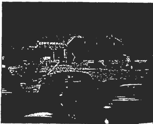
Figure 4-4: Metal structures being constructed at TA-21 DP West, Post War Era (circa 1945)
